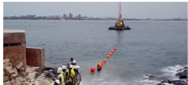
Figure 3. Installation of the 2.7 km submarine power cable connecting Gorée Island to Dakar’s grid, replacing diesel generators, and improving energy security (Source: World Bank, 2018).
